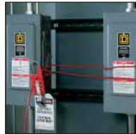
Lockout single or multiple electrical disconnects
