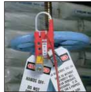
Lockout gate valves
