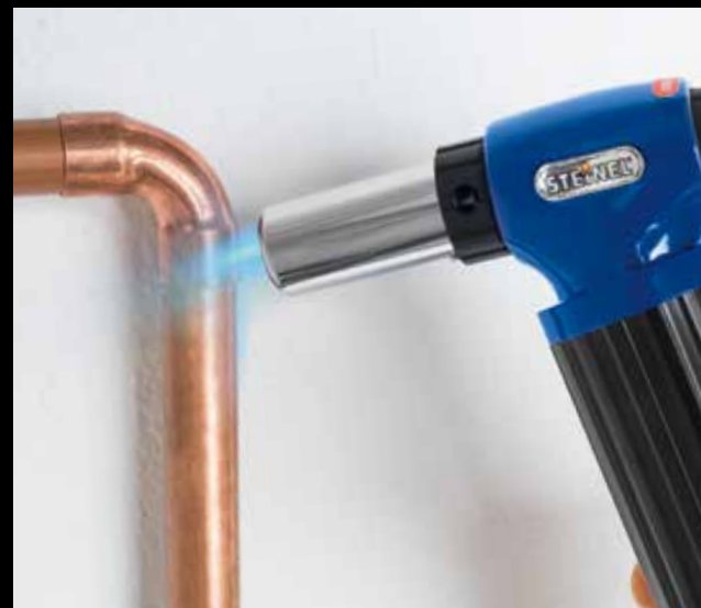
Solder joints on copper piping
